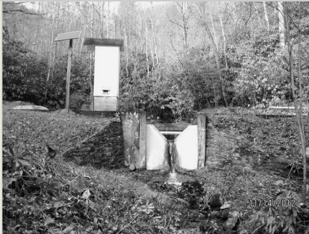
Figure 3.1 Upstream view of 90° V-notch weir installation on WS 7, November 2012.
